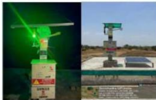
Pilot Project Lightning Early Warning System at Sonbhadra
